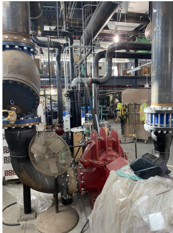
Chilled Water Pumps in Mechanical Room
